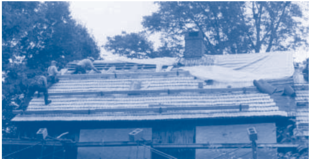
Historic materials were protected with plywood panels as the Morgan Log House got a new roof. The wood shingles precisely replicated ones made in the 1700s.
